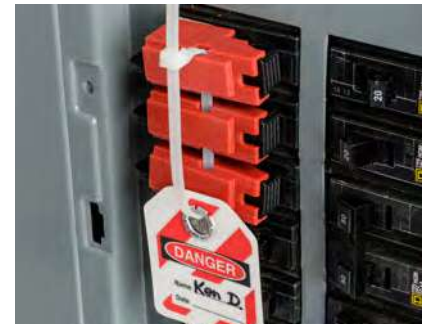
120V breaker lockout devices fit on breakers next to each other, enabling multiple tagouts at one time
