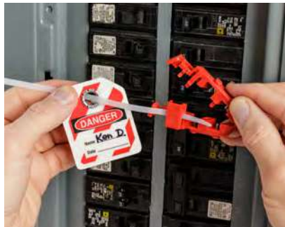
Save time by “pre-loading” your tag and cable tie before walking to the energy point
